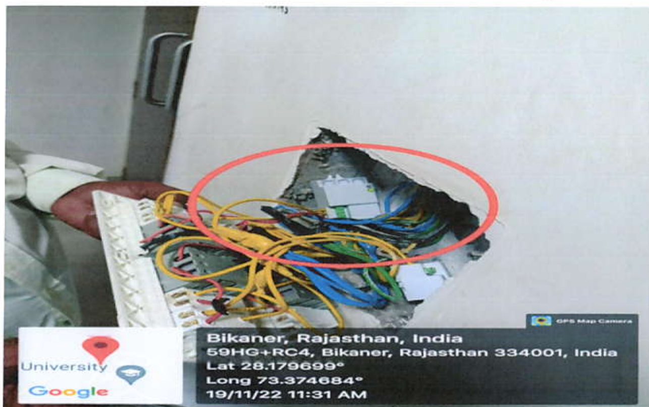
Motion Sensors Installed in Switch Boards of Academic Block
