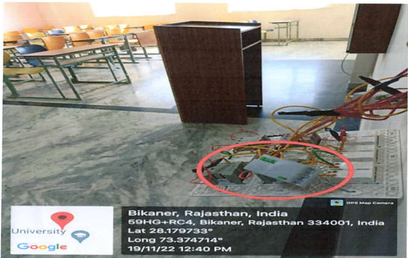
Sensor installed in Switch Board for Energy Conservation
