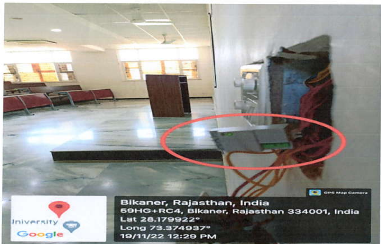
Sensor installed in Switch Boards of Academic Building Class Rooms
