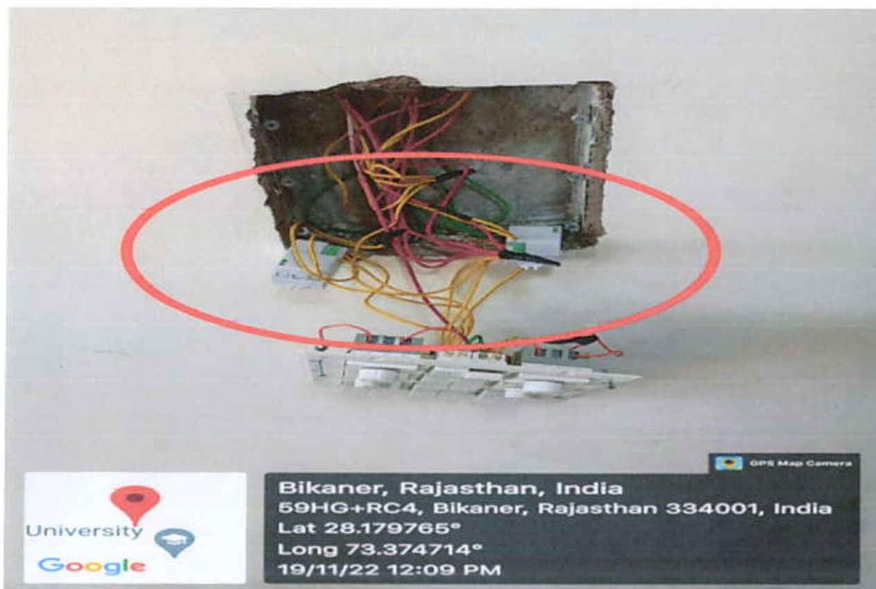
Motion Sensors Installed in Switch Boards of Admin Building
