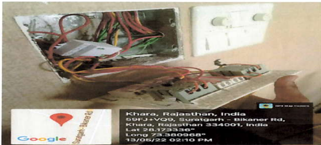
Sensor Installed in Switch Board for Sensor Based Conservation
