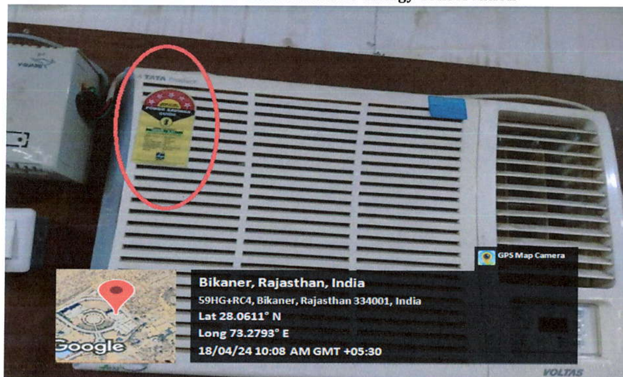
Five Star Rated AC Installed for Energy Conservation
