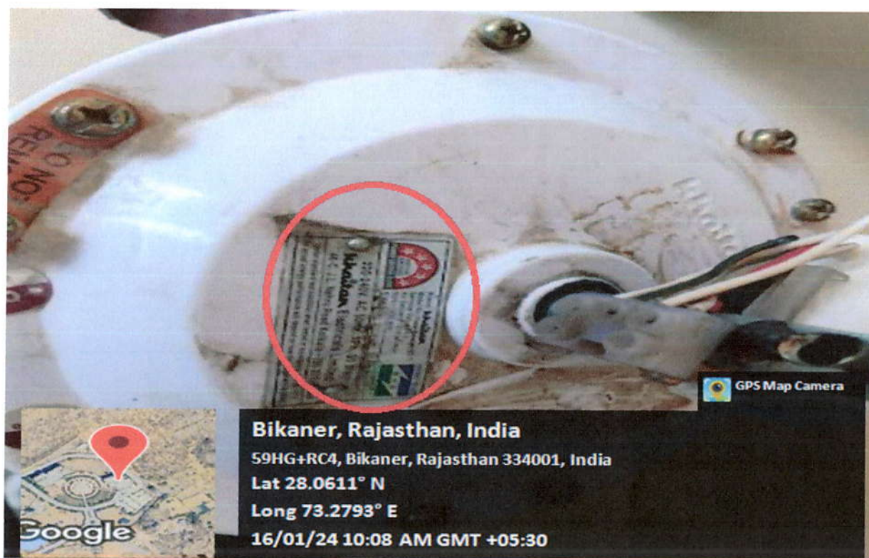
Five Star Rated Fans Installed for Energy Conservation
