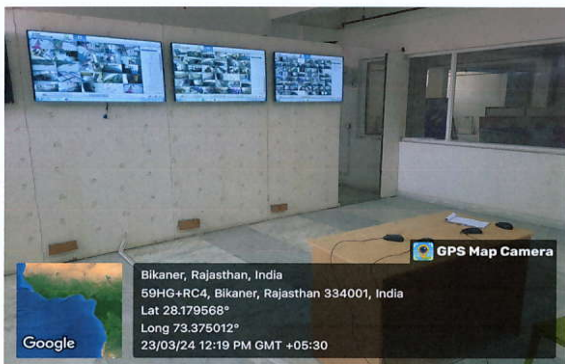
CCTV Control Room of RNBGU
