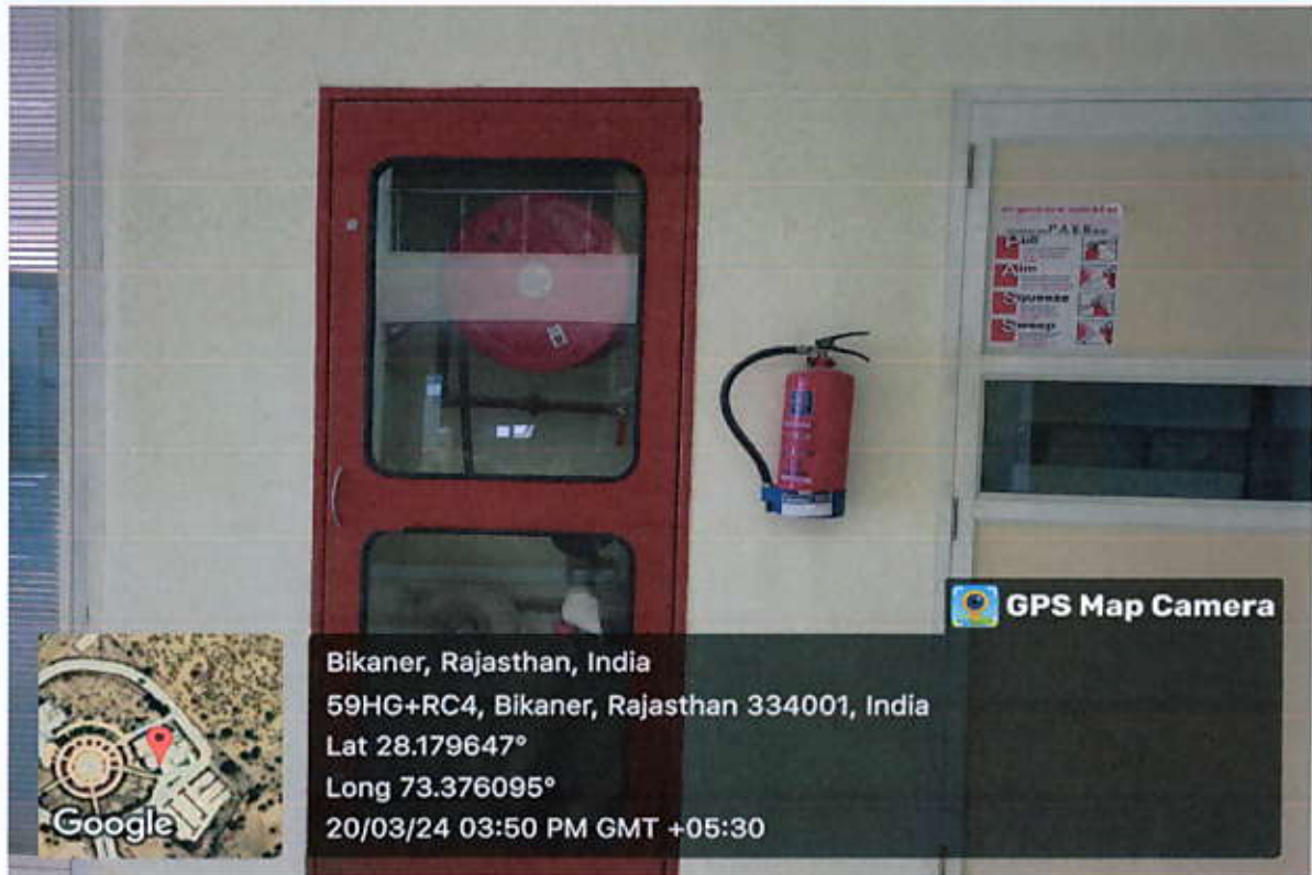
Water Hydrants and Fire Extinguisher in Academics Block
