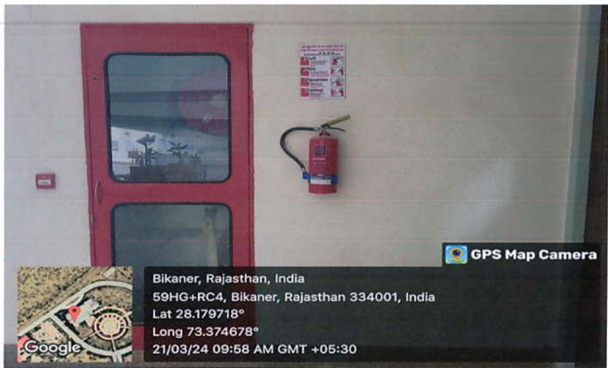
Water Hydrants and Fire Extinguisher in Admin Block
