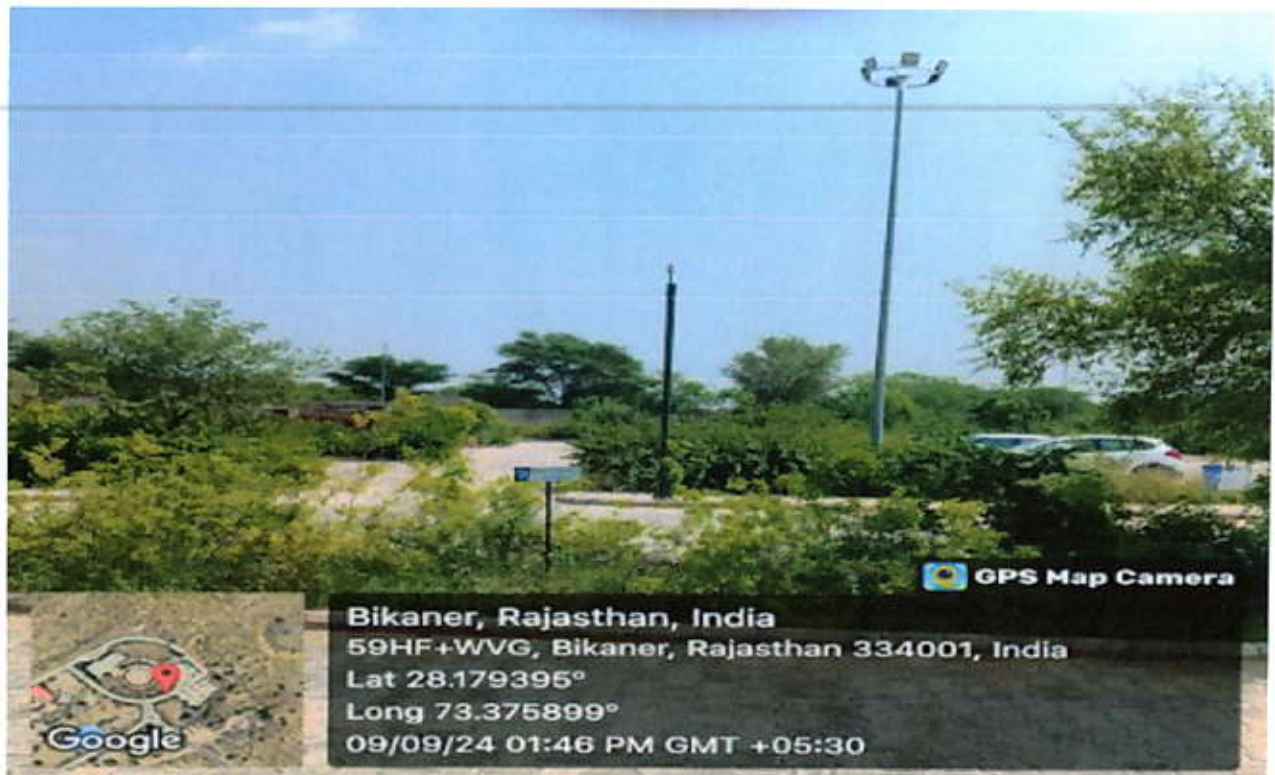
High Mast Lights
