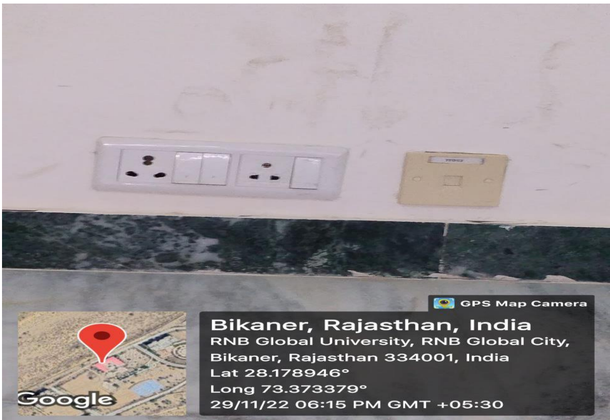
Third Floor Room No. – 311 Inside- LAN Socket
