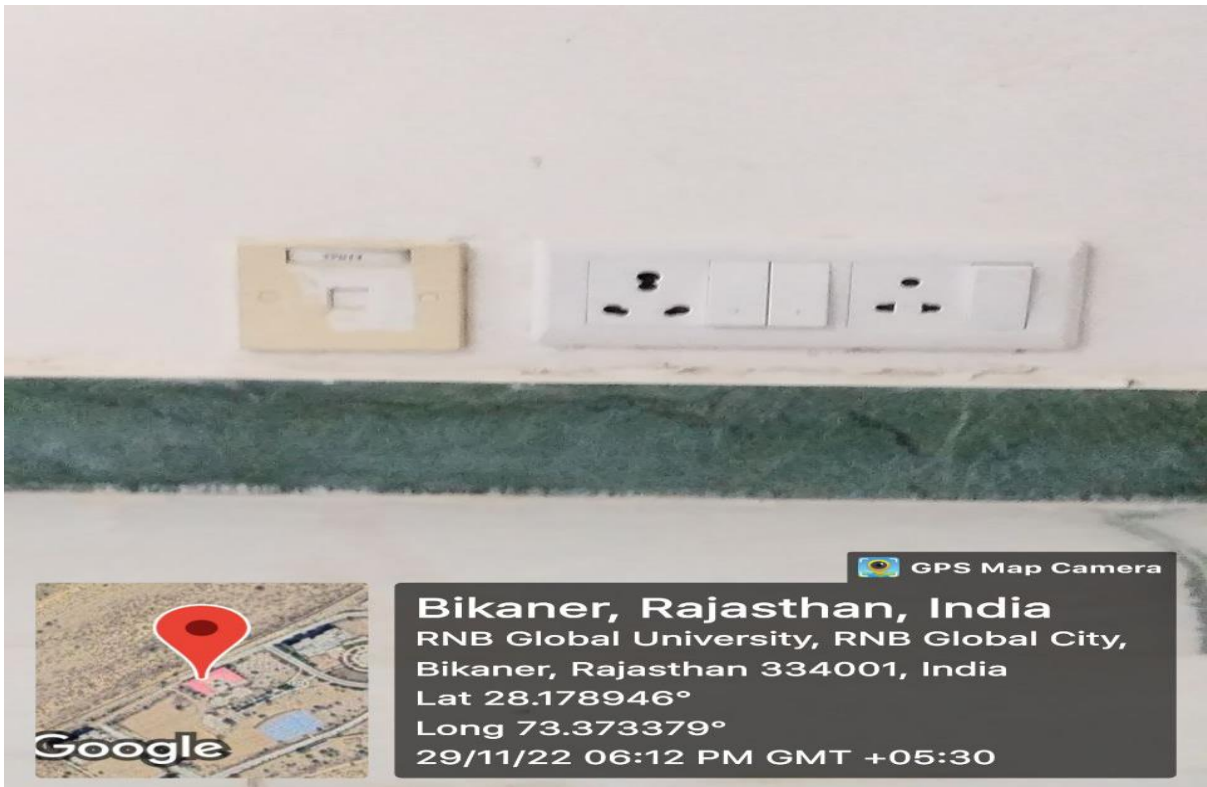
Third Floor Tutorial Room No. - 310 Inside LAN Socket
