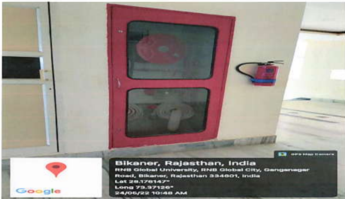
Fire Safety- Administrative Block
