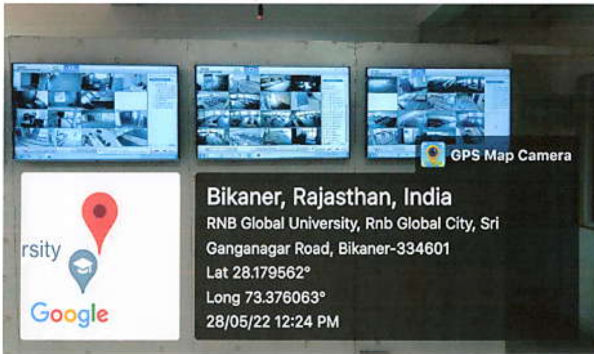
CCTV Control Room
